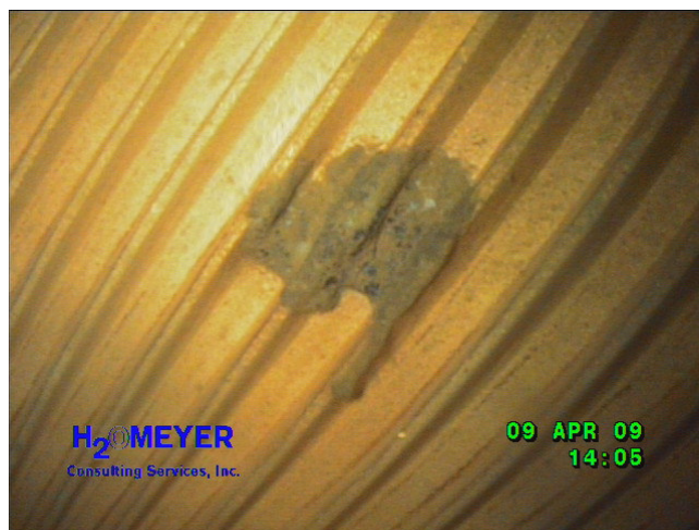
Row 30, Tube 41 – Some visible corrosion.
