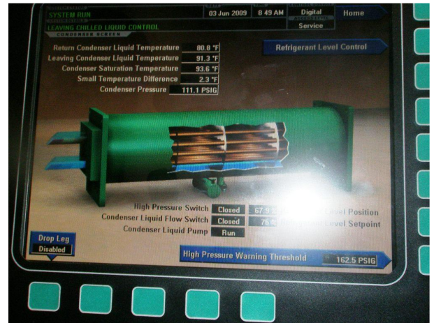
Figure 1: Many newer Chillers have approach temperatures already displayed.
